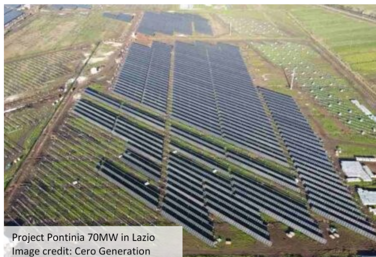
Figure 40 Cero Generation's 70 MW Pontinia project in Lazio
